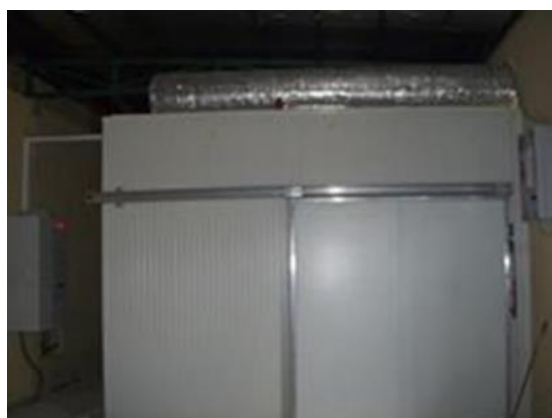
Figure 1. Cold store general view
