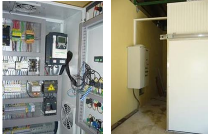
Figure 3. Electrical control box of the cold store
